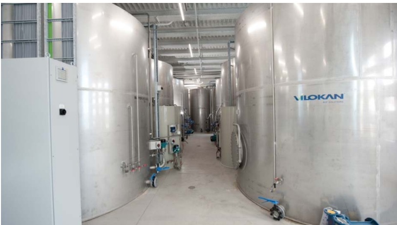
Step 4 – cont'd Quality-control tanks.
